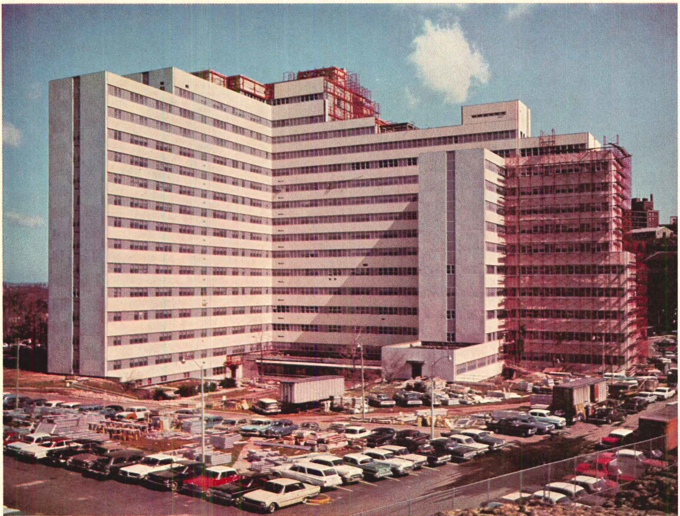
Over one million bricks were replaced by Plasteel aluminum panels while the hospital continued its day-to-day operation.
