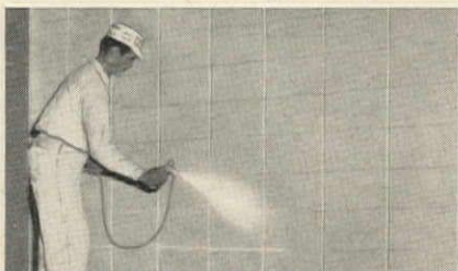
Final coat sprayed in colors. Within 48 hours, first coats were inspected and touched up. The final coat, in six different shades, was applied with airless sprayers. Beige, light beige, blue, carrot, dusty gray, and "incense" were used.
