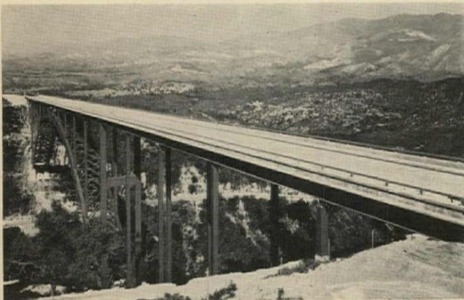
Category: Best Design and Engineering in Public Works Construction—Cold Spring Canyon Bridge, Bridge Department, Division of Highways, State of California Designer: Marvin A. Shulman Resident engineer: Fred H. Yoshino General contractor: American Bridge Division, United States Steel Corporation
