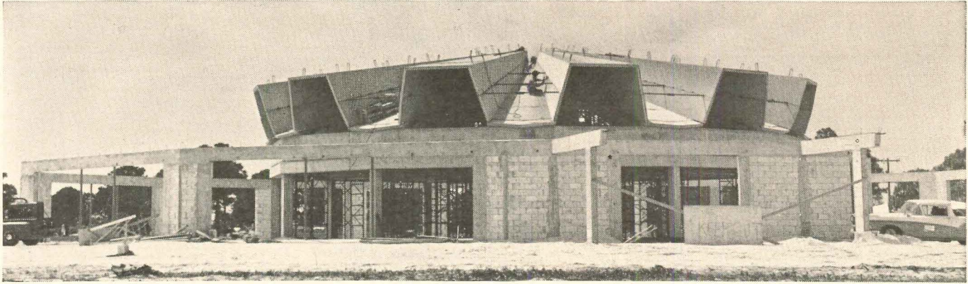
At St. Ambrose School and Provisional Roman Catholic Church, schoolrooms surround the religious area which is located under
