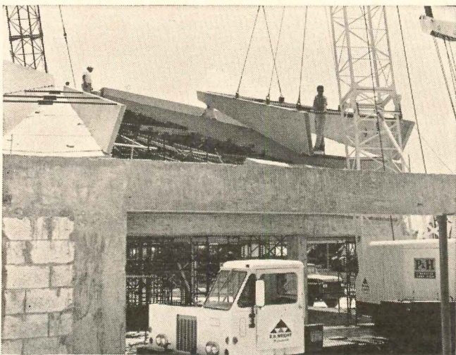
(LEFT PHOTO) Placing one of the 36' long precast concrete tapered folded plates. Only two days were required to place the 24 roof units. (RIGHT PHOTO) Deep folded plate design is
