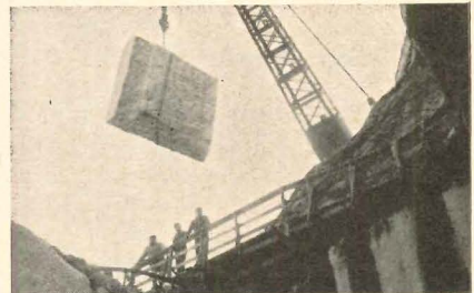
Outsize blocks of marble were taken from our Danby quarry for this installation. 250 slabs with random, non-matched veining were specified by architects Skidmore, Owings & Merrill.
