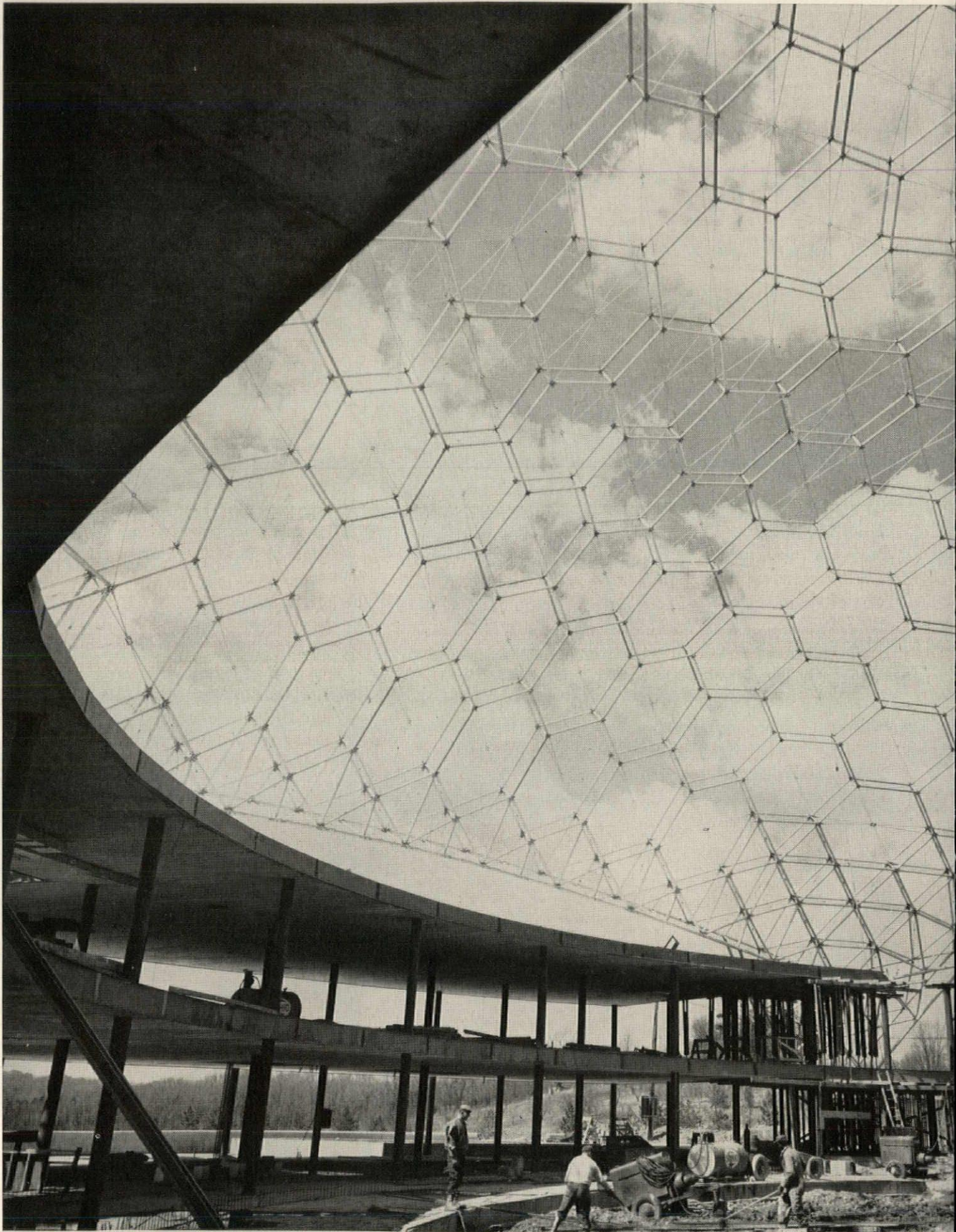
Owner: The American Society for Metals / General Contractor: The Gillmore-Olson Company, Cleveland, Ohio / Architect: John Terence Kelly, Cleveland, Ohio / Dome Design: Synergetics, Inc., Raleigh, North Carolina / Aluminum Materials: Kaiser Aluminum & Chemical Sales, Inc.
