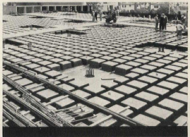
Ceco's one-piece Steeldomes in position, ready for reinforcing steel. Easily erected and removed, Steeldomes speed construction. There is no excessive clean-up expense because forms fit tight, leave no unsightly residue.
