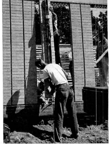
"SCR building panels," each made up of thirty-six norman-face brick set in stacked bond, are vacuum-lifted into place
