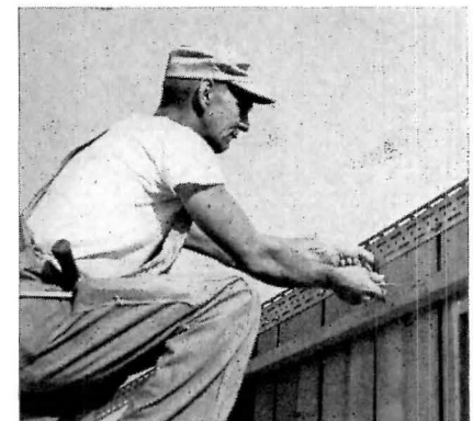
A single bolt at top and bottom of each panel secures them to horizontal steel angles attached to the sills
