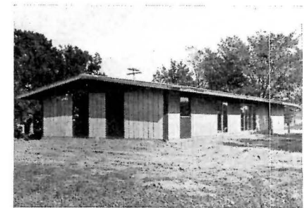
The brickwork completed — by five men in eight and a half hours, roof trusses are installed and finishing work begun
