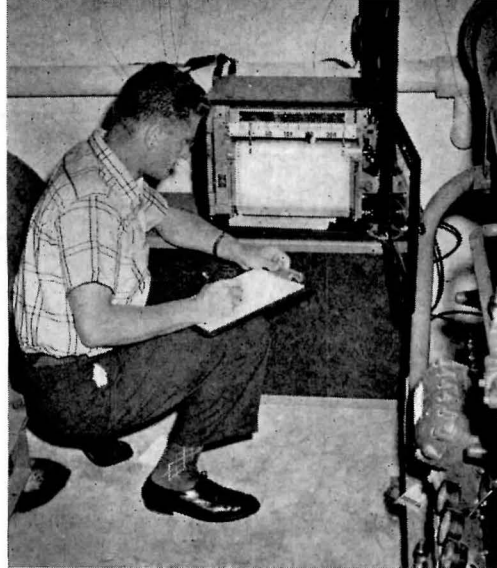
At left, the pyroheliometer is being installed inside a south window to measure solar radiation. At right, a recording potentiometer charts the supply and return chilled water temperatures
