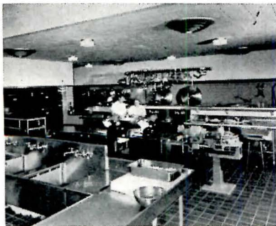
Vegetable and potato preparation area in South Quadrangle, University of Michigan. Kettles, steam cookers in background; ovens left. Air diffusers in ceiling
