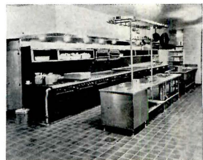
Ranges, grills and fryers are in one line behind ovens, also under exhaust hood. Tile floor is well supplied with drains
