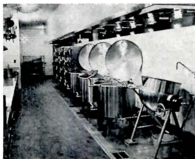
Closer view of kettles and steam cookers shows removable drains in stainless steel gutter and powerful furred-in exhaust hood above
