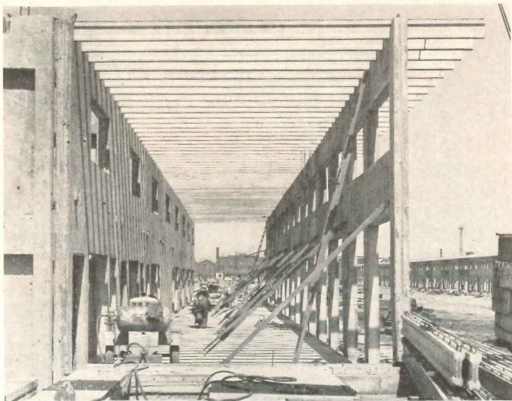
Looking down through the con- course area on the truck side. Panels are connected by precast joists
