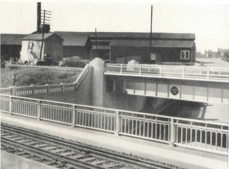
Railings of Alcoa Aluminum on this Little Rock, Ark., railroad bridge have stood up through fifteen years of smoke and soot; never needed paint or upkeep.
