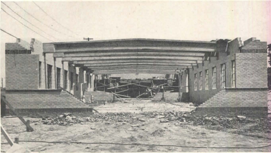
Above: prestressed roof beams for machine shop of geophysical laboratory in Tulsa, Okla. Beams were prestressed with 14, 1/4-in. high-carbon wires. Below: ceiling of main laboratory building; 30-ft beams are prestressed, girders are not
