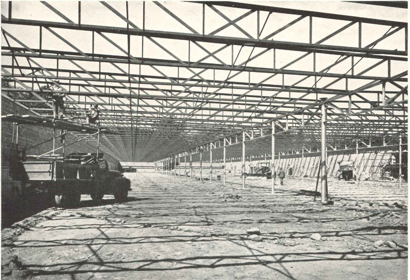
Installation of Bethlehem Longspan Joists in Fernbrook Park Mill (Dallas, Pa.) of Bloomsburg Mills, Inc. Architect: Lacy, Atherton and Davis, Wilkes-Barre, Pa. Contractor: Sordoni Construction Co., Forty Fort, Pa.
