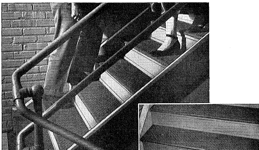
Photograph of Feralun Safety Treads installed in the office building of the RCA Victor Division, Camden, N. J., when the building was erected in 1923. (Photo courtesy Public Relations Department, RCA Victor).
