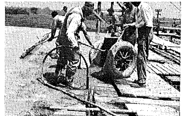
Concrete is being poured here over the steelforms and around the reinforcing steel. The final step is removal of steelforms and lumber after concrete sets.
