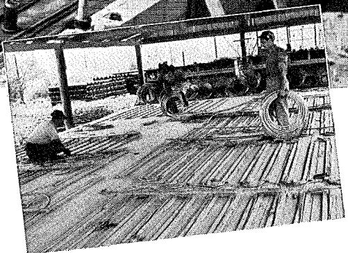
TO SAVE TIME AND MONEY IN HANDLING and installing the radiant panels for heating, the Revere Copper Water Tube was speedily bent into wooden forms by hand, then wired to temporary frames and stacked flat until needed. Tube sizes run from ¾" to 1¼".
