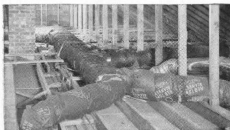
Attic view shows insulated supply ducts that connect via warm-air inlet boots to the ceiling panels below. Sealed insulation board is used to form top of ceiling plenum. Uninsulated pipe at right is exhaust for kitchen ventilating, not connected with heating system. Photograph taken before insulation was installed between joists.
