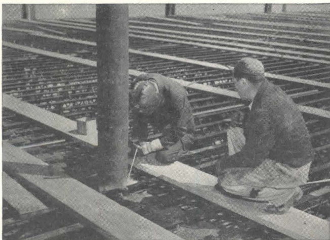
Fig. 1. Welding pipe column to first floor I beam. Column has a smaller pipe and concrete inside.
