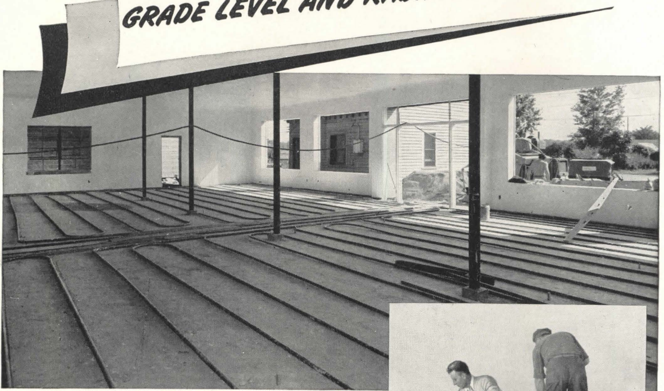
Radiant Heating Coils resting on Zonolite Insulating Concrete
