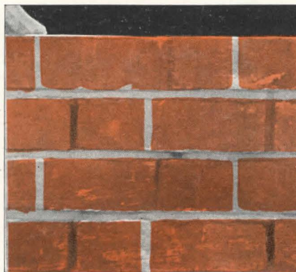
This encourages the bricklayer to fill the head joints, since proper tooling cannot be done if mortar is lacking.
