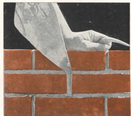
Therefore before the tooling can be completed, it is necessary for the bricklayer to point up the open joints.
