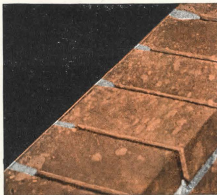
there is very little mortar in the cross joint.
