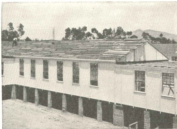
Cemesto walls on one of the sections of the large Naval Hospital at Corona, Calif.
