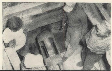
(Left) Normal traffic was maintained on this busy downtown street while Ric-wil units were installed under pavement. Units were jacked through from building basements and joined to utility's steam main at manhole in center of street. (Right) Close-up of manhole showing auger crew and tool for drilling under pavement.
