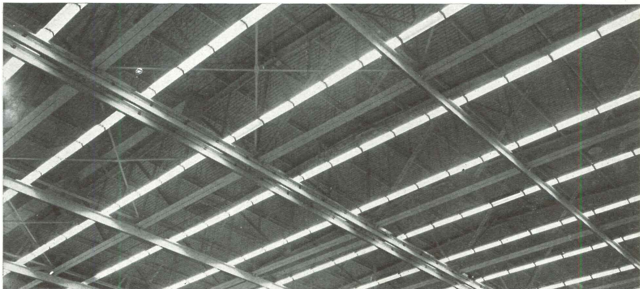
Above, fluorescent lighting in a monitored daylight plant. In the near future, fluorescent will have to compete with cold cathode. Below, lights in a complete "blackout" plant, giving full control and low maintenance but raising questions of effect
