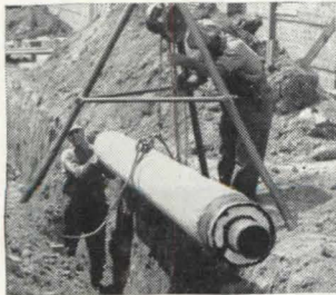
Section of Ric-wil prefabricated insulated steam conduit being lowered into shallow trench for steam connection to a new apartment at Shaker Square.
