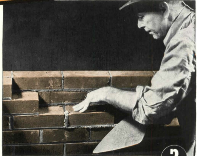
(1), it is much easier to shove the brick accurately into place, with a full head-joint, than it is to do the same thing with the other mortar (2).
