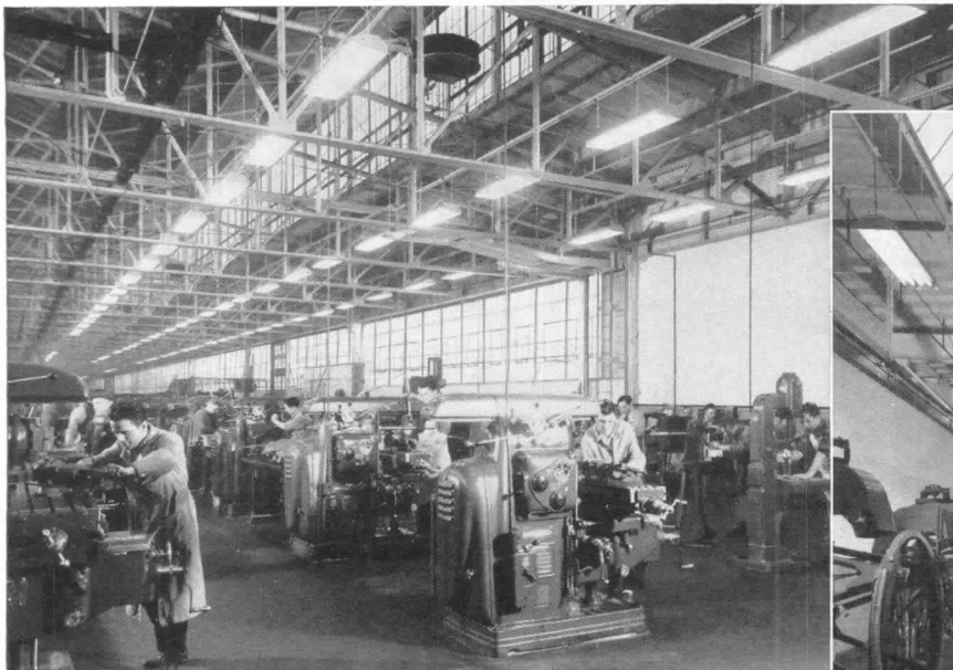
Trim, overhead mounted Trane Projection Unit Heaters contribute to the efficient appearance of the plant.
