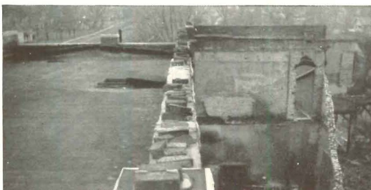
Although the low fire wall of the bank offered little protection, the flames were stopped by the J-M Asbestos Roof.
