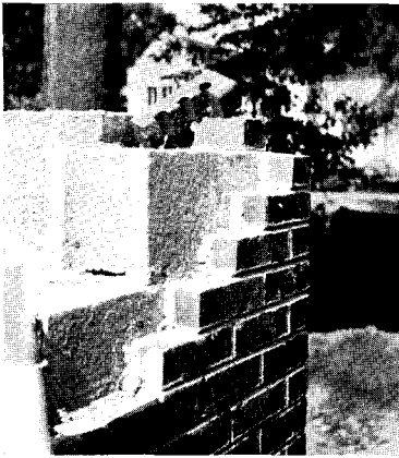
Fig. 26. Brick-faced concrete masonry using split brick. A saving in construction cost results from smaller quantity of face brick required.
