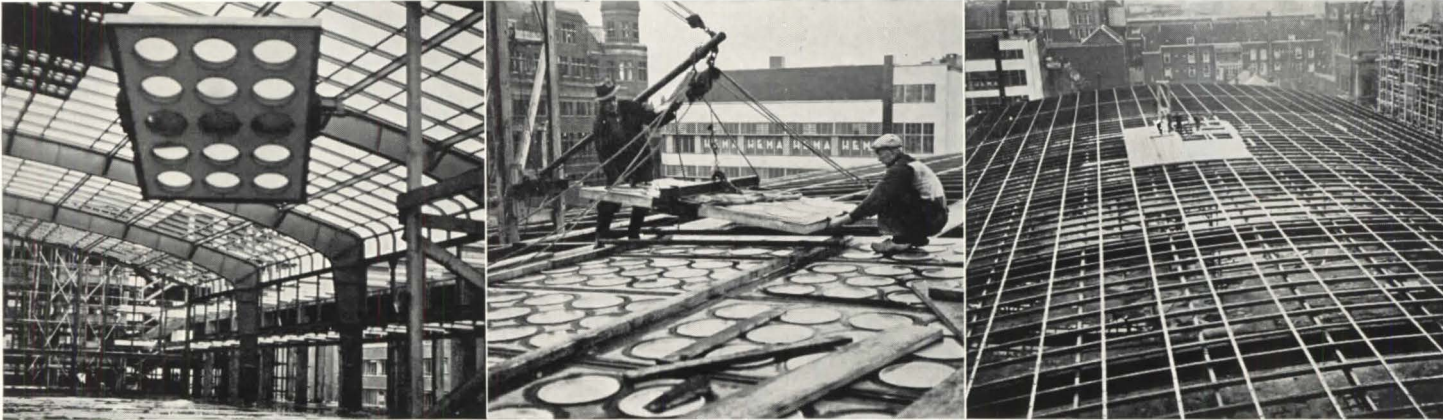
Glass-crete units are raised to roof . . . projecting ribs fit into U-shaped purlins . . . which run between welded arched girders.
