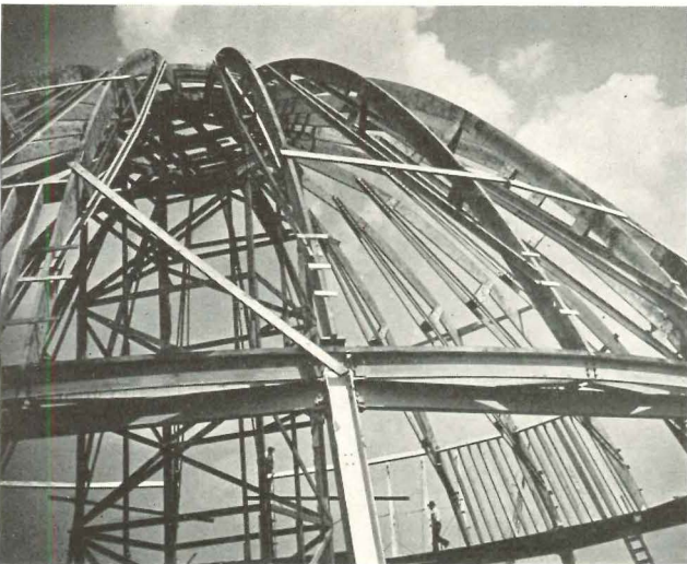
Wood templates in place on dome of Distilled Spirits Building, timber studding follows.
