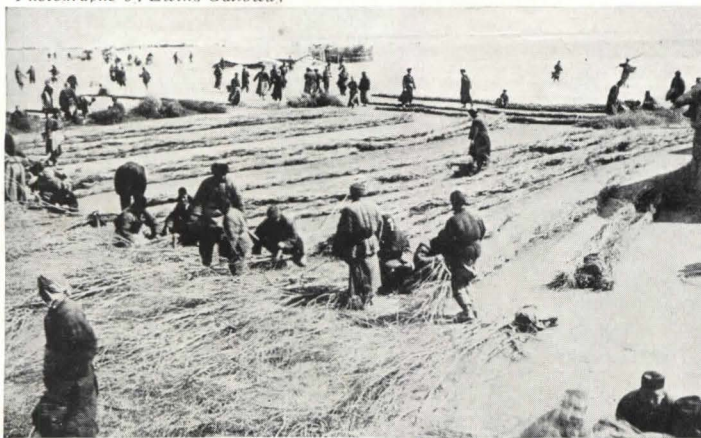
MORE THAN 5,000 TONS OF HEMP and tens of thousands of willow branches were used in making fascines to build a 600-mile dike. The branches are laid out in straight rows 50 feet long along the ground, twisted together and then tied with hemp rope.
