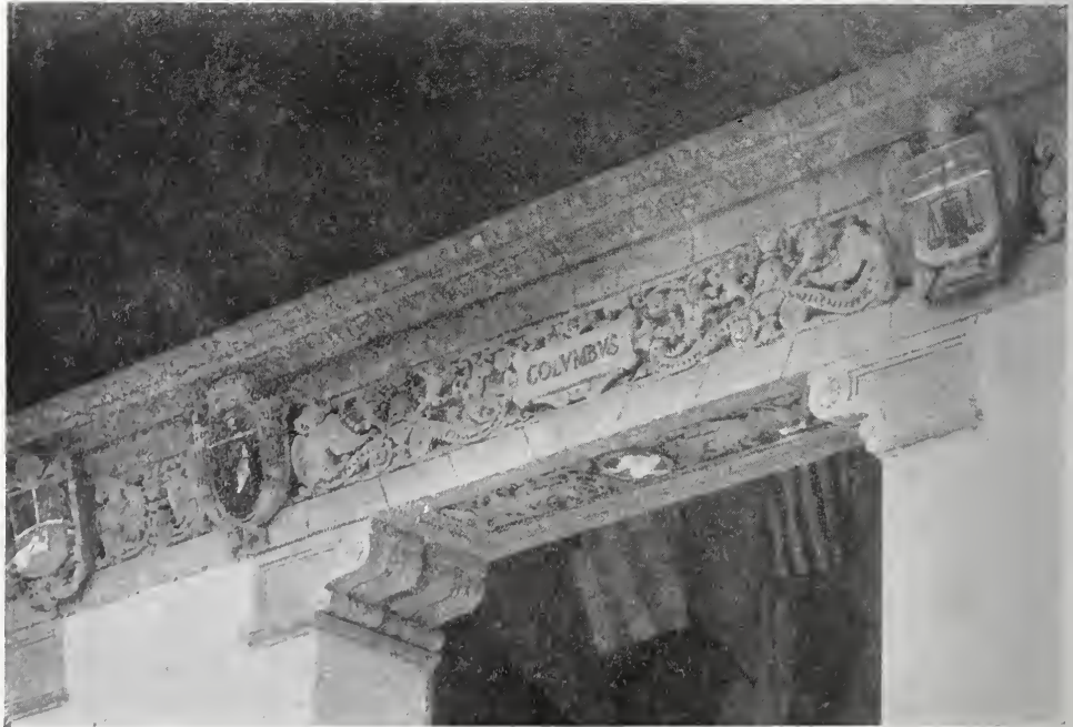
DETAIL OF POLYCHROME TERRA COTTA FRIEZE AND SOFFIT IN THE PATIO, THE PAN-AMERICAN BUILDING, WASHINGTON, D. C.
