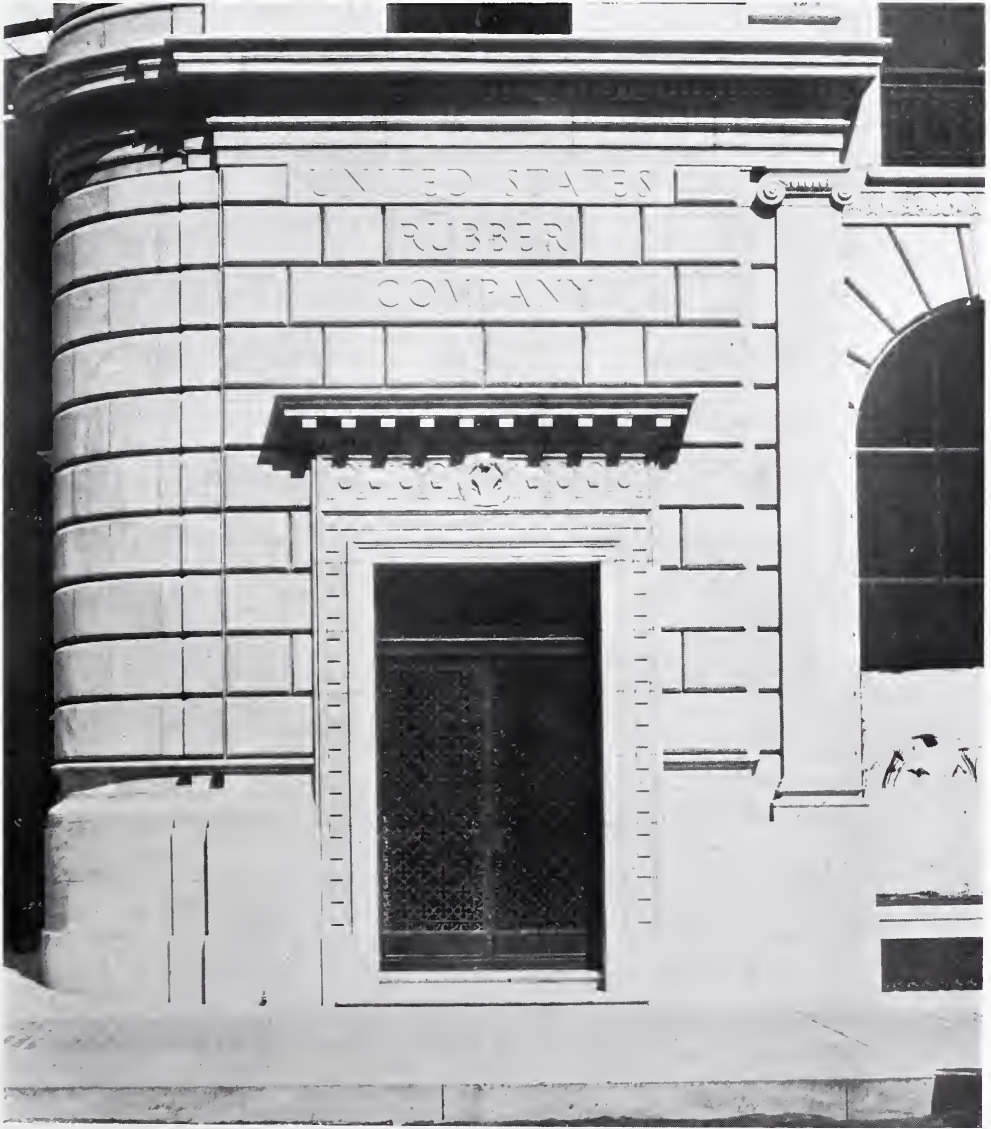
ENTRANCE DETAIL. BUILDING FOR THE UNITED STATES RUBBER COMPANY. Carrère and Hastings, Architects.
