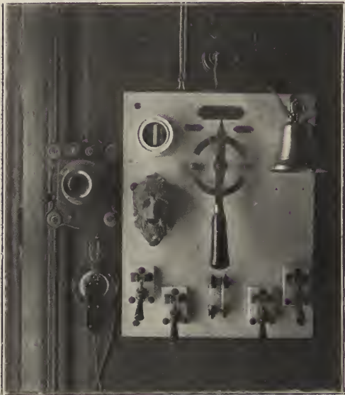
VILLA FERIA ELECTRA—TELEPHONE AND PLAQUE COMMUNICATING WITH THE ELECTRIC GATE.
