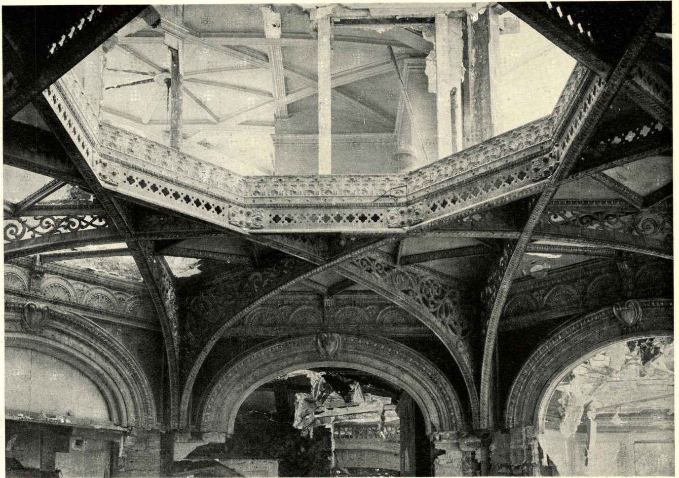
THE OPEN WELL of the main hall, in structural and decorative cast iron, shows how closely the decorative scheme was made to follow construction
