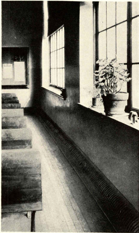
A register runs the entire width of the exterior wall of each class room. Exhaust vents are on the facing wall
