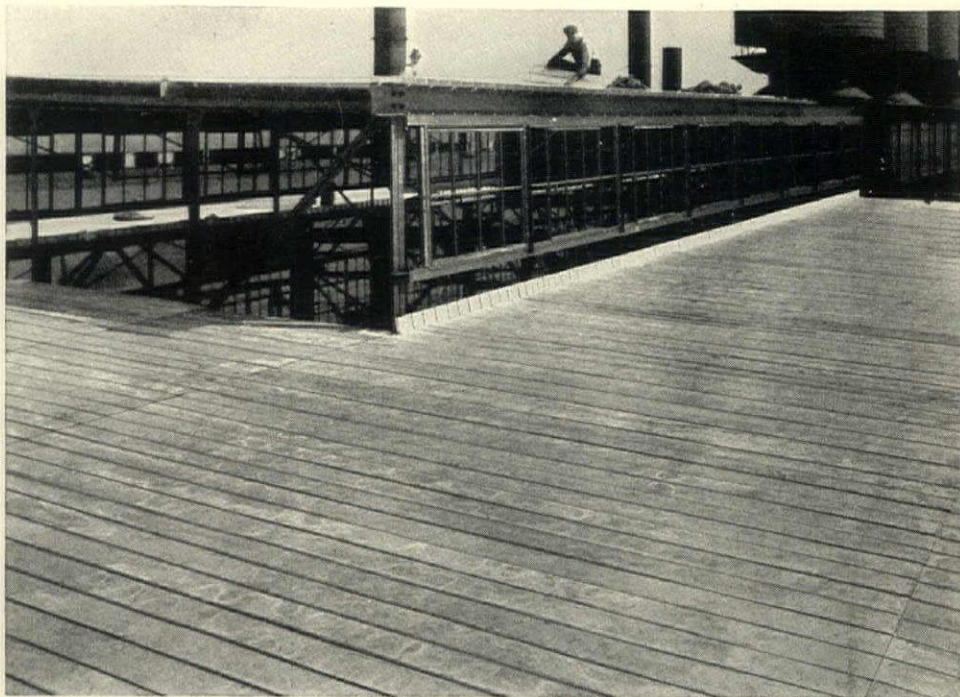
Mahon Steel Roof Deck installed on a new plant for the Latrobe Electric Steel Company, Latrobe, Pa.
