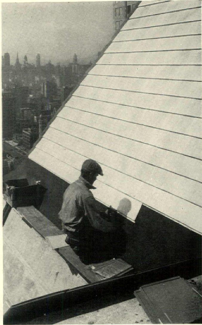
Aluminum shingles being applied to the annex of the Drake Hotel, Chicago. Benjamin H. Marshall, architect
