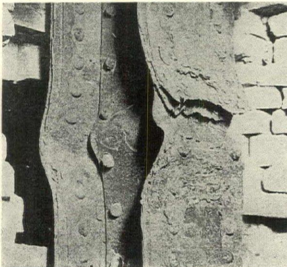
Detail of a steel column which was carried through a boiler wall between two fireboxes in a Detroit building. The column was too close to the heat and corrosive gases, with the result shown. Eleven years ago it was reinforced due to the same causes. Now it is being removed entirely and the upper portion will be carried by girders above the boilers
