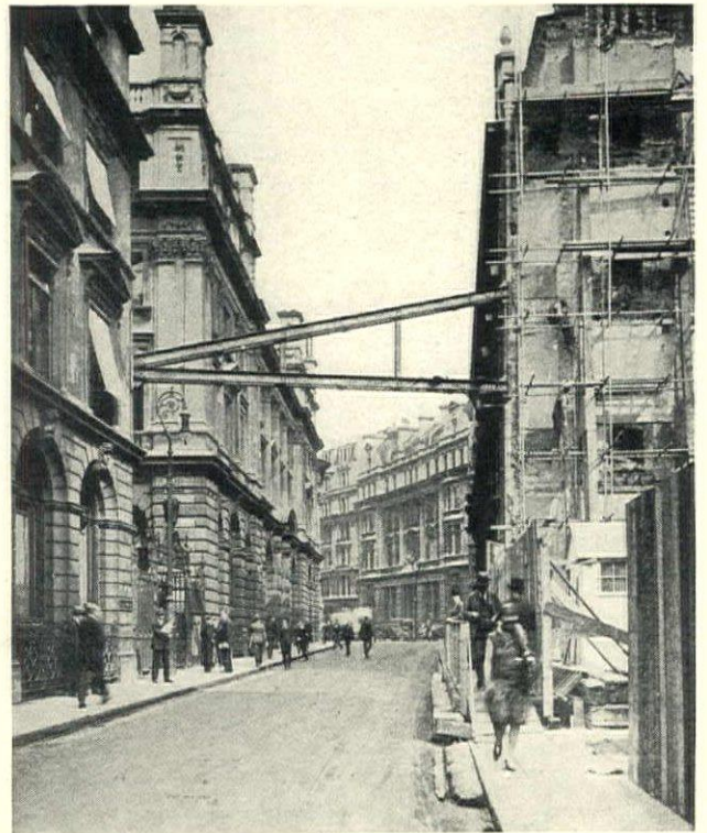
This steel girder is said to be the first used as a shore across a main thoroughfare. It is about thirty feet above the level of the pavement. Threadneedle Street, London, England
