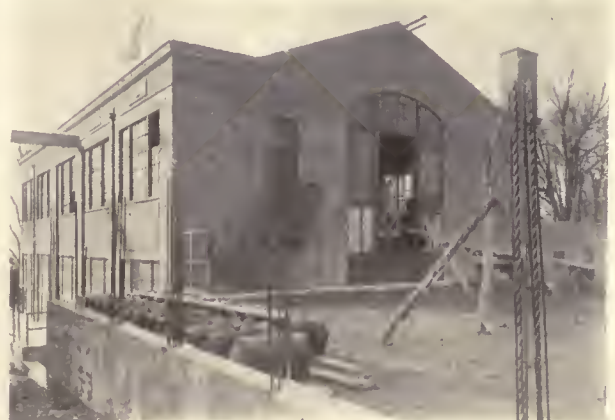
REAR ELEVATION. NOTE HOISTING BEAM AND LARGE OPENING OF OPERATING ROOM FOR PLACING EQUIPMENT
