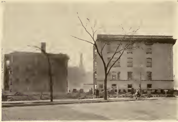
TURNING OF SECTION 2 ALMOST COMPLETED AND READY TO BE MOVED BACK INTO FINAL POSITION. SECTION 1 AT LEFT AND UNDERPINNED WITH BRICK ON NEW FOUNDATIONS. SECTION 2 STILL IN IRVING AVENUE, JACKSON BOULEVARD IN FOREGROUND.
