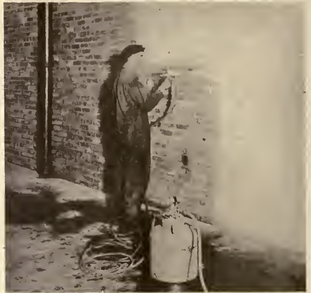
IMPROVING THE APPEARANCE OF A COMMON BRICK FACTORY WALL
