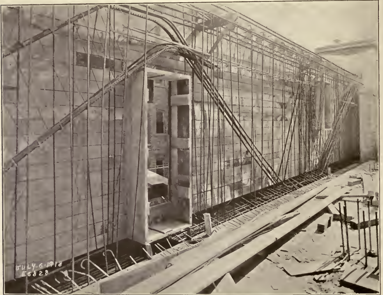
PHOTOGRAPH ILLUSTRATING METHOD OF PLACING REINFORCEMENT FOR REINFORCED CONCRETE TRUSS SO AS TO ALLOW FOR THE TWO OPENINGS
