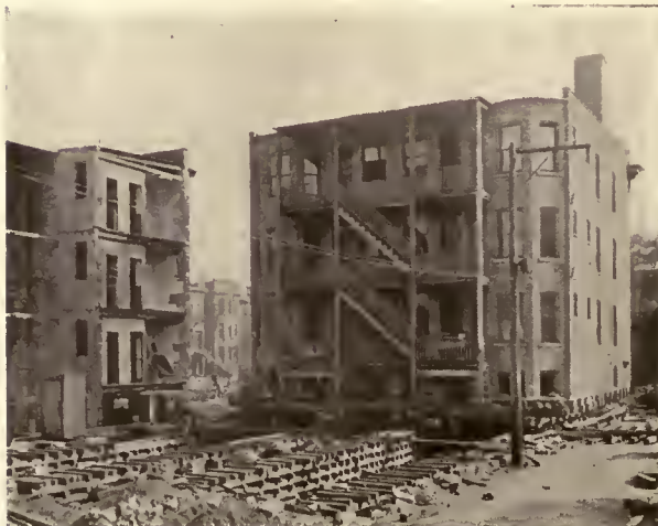
REAR OF SECTION 1 LOOKING EAST. THE BUILDING IS MOVED INTO IRVING AVENUE AND READY TO BE TURNED 180 DEG. ON ITS CENTER. TO THE LEFT IS REAR OF SECTION 2. NOTE THE SILLS, ROLLERS AND CRIBBING.
