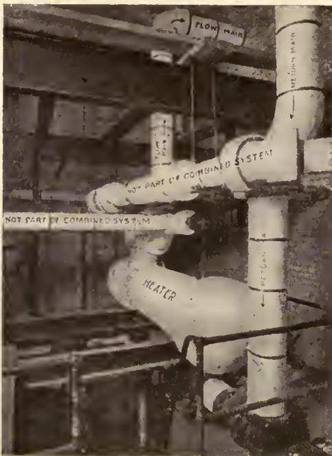
GENERAL VIEW OF HEATER ROOM. NOTE SIMPLICITY OF ARRANGEMENT
