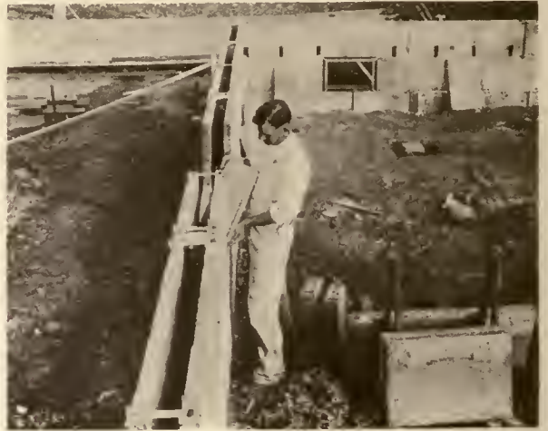
CONSTRUCTING A DOUBLE WALL WITH CONCRETE BLOCKS. IN THIS CASE THE AIR SPACE IS CONTINUOUS AND FURRING THE INTERIOR IS UNNECESSARY
