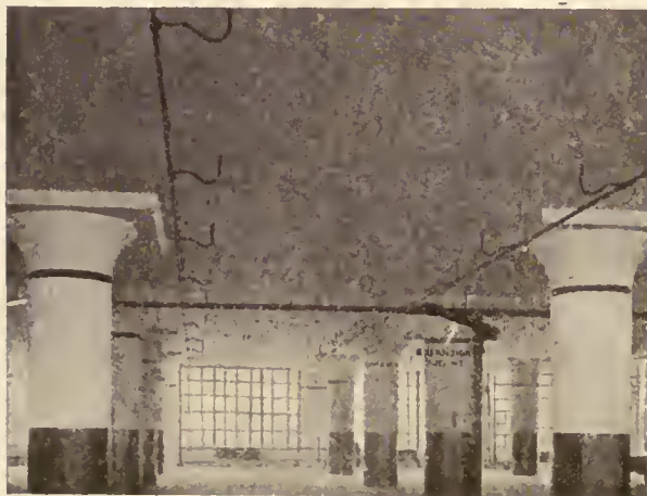
GENERAL VIEW OF SPRINKLER LINES. INSULATING ARMS AND EXPANSION JOINT CAN BE SEEN
