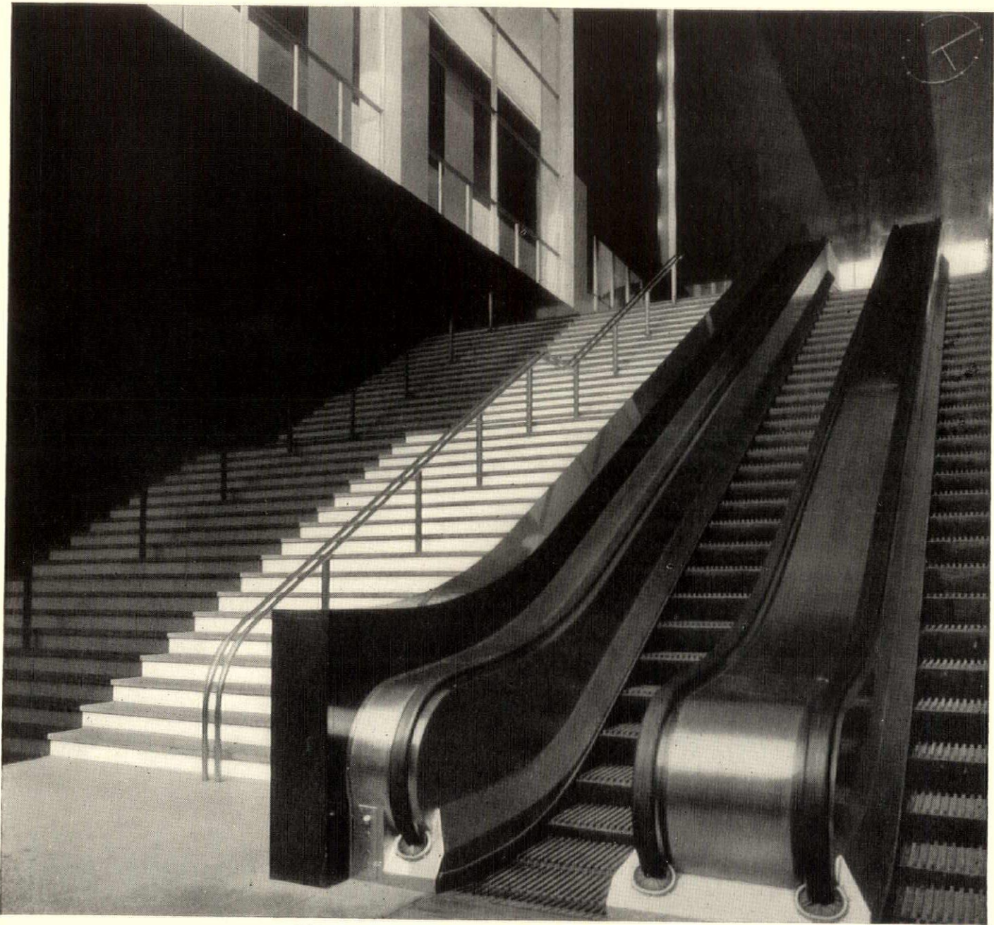
Photograph of escalators in the new building of The Philadelphia Saving Fund Society
