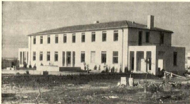
A new dormitory and dining-hall for the American Junior College, Ellenico, Greece, now under construction. Thompson & Churchill, architects, of New York
