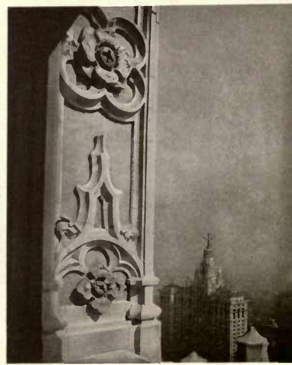
DETAIL OF WINDOW-JAMB, WOOLWORTH BUILDING, NEW YORK. Cass Gilbert, Architect. Polychrome terra-cotta.
