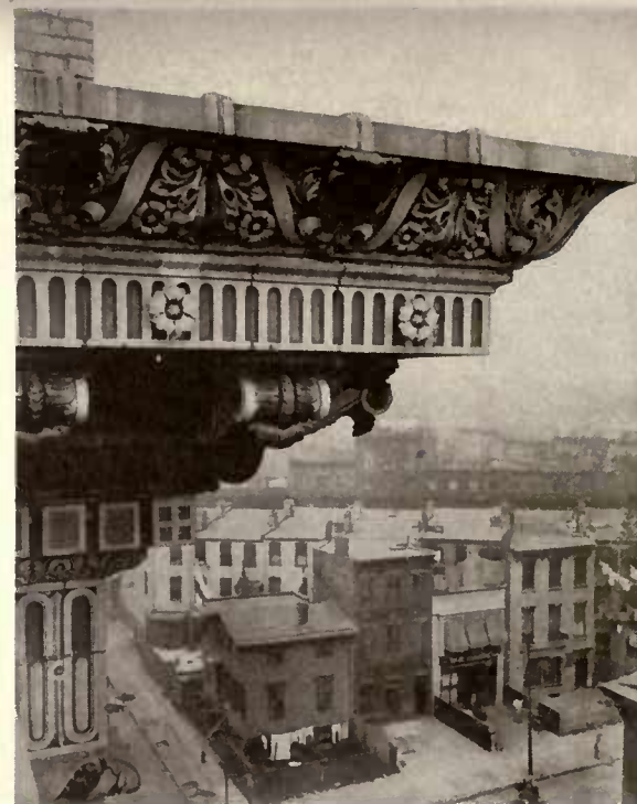
BROOKLYN ACADEMY OF MUSIC. Herts & Tallant, Architects. Section of main cornice of polychrome terra-cotta.
