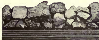
Actual photograph of a cross-section of a Barrett Specification Roof. Note the uniform distribution of Specification Pitch between the layers of Felt.
