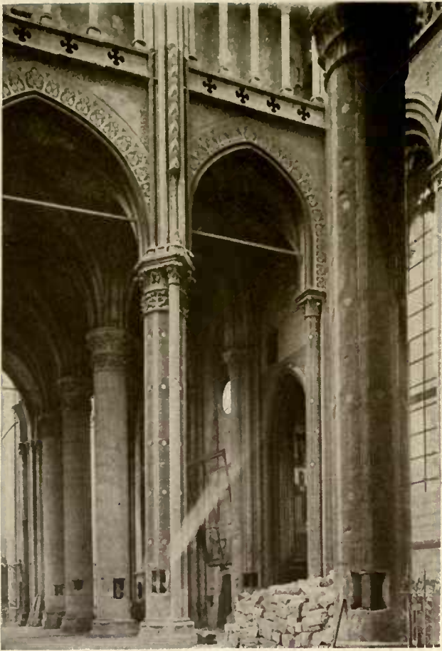
St. Quentin (Aisne), April 23, 1919. Showing piers drilled for mine by Germans. To the right the frame of a painting which has been cut out and carried away.
