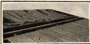
Upper half of roof is ordinary steel. Lower half is “Copmetl.” They are of same gauge and were laid simultaneously.
