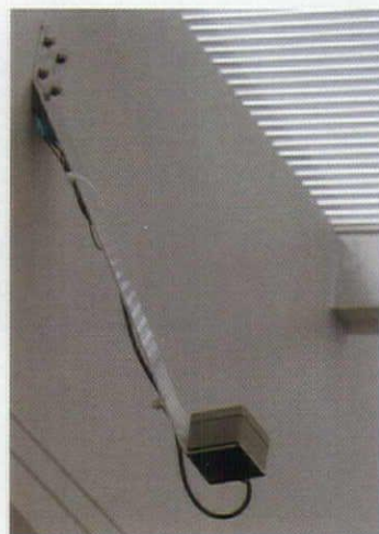
For the small percentage of time when a K-12 facility might operate outside of daylight hours, a high-efficiency luminaire is integrated into the skylight / halo system. Ceiling fans provide air circulation to aid in overall cooling (left). The light sensor (above) adjusts the louvers to maintain an overall light level of between 20 to 40 footcandles throughout the classroom.
