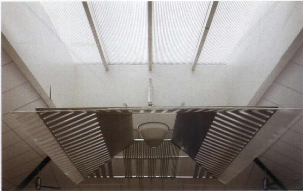
The key components of the Mount Angel high-performance classroom prototype are a skylight with automatically adjusting louvers and a specially designed apparatus called the "halo," which hangs below and helps reflect light (above). Throughout the testing period, the mockup functioned as both a working lab and a classroom (below). Seen from directly below, the skylight and halo have a sculptural quality (facing page).
