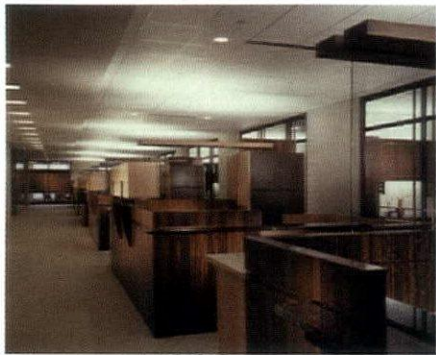
Top: Ground-based permanently installed indirect fixture. Bottom: Fixed-mounted direct/indirect fixture with modular layout. Walls move around fixtures, sprinklers and air diffusers.
