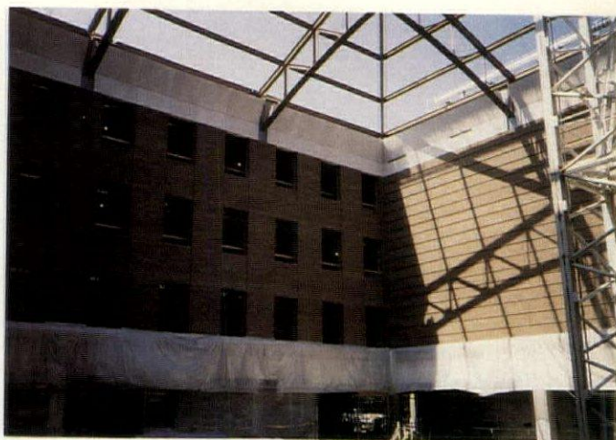
The new University of Michigan chemistry building under construction at Ann Arbor.
