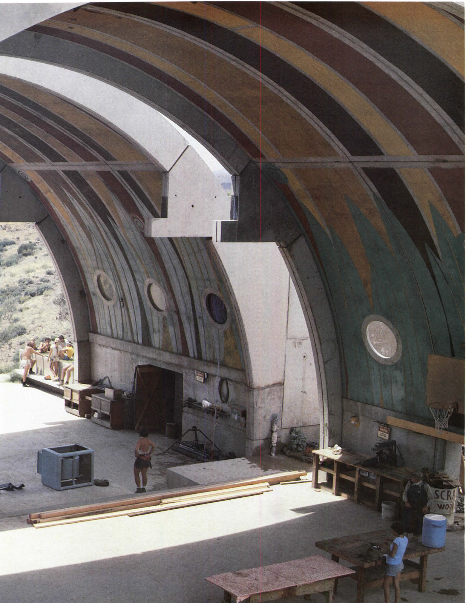
The north and south vaults where breakfast and lunch buffet occur, also containing the weld shop and electrical shop.
