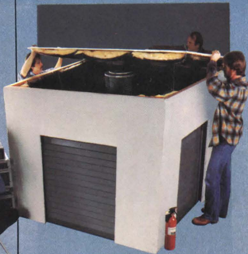
Actual installation of Cookson rolling doors—sensitive equipment is protected in this defense facility.
