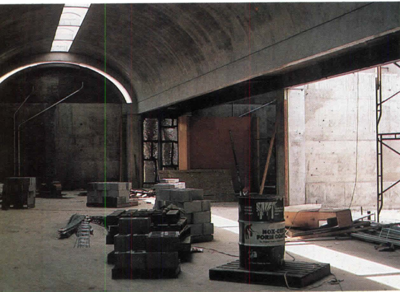
Kimbell before and after the reflectors (left). Below, a section incorporating reflectors.
