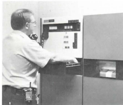
Chief of Plant Operations, Sterling Clarke, runs daily status check of all building utilities through this Master Control Panel.
