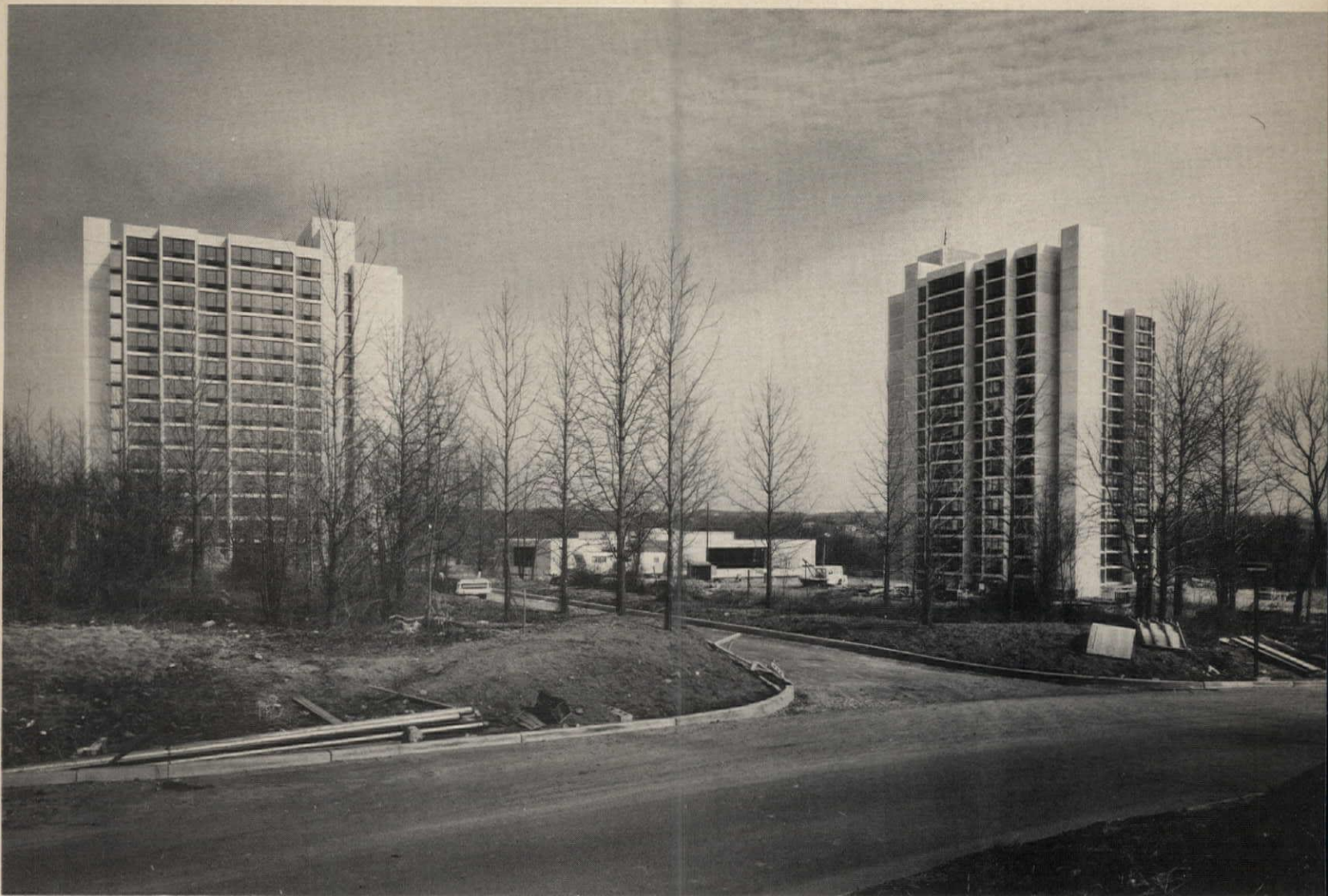
The $10.5 million center is about completed, a year after the pouring of foundations began. The towers went up at a rate of one floor a week.
