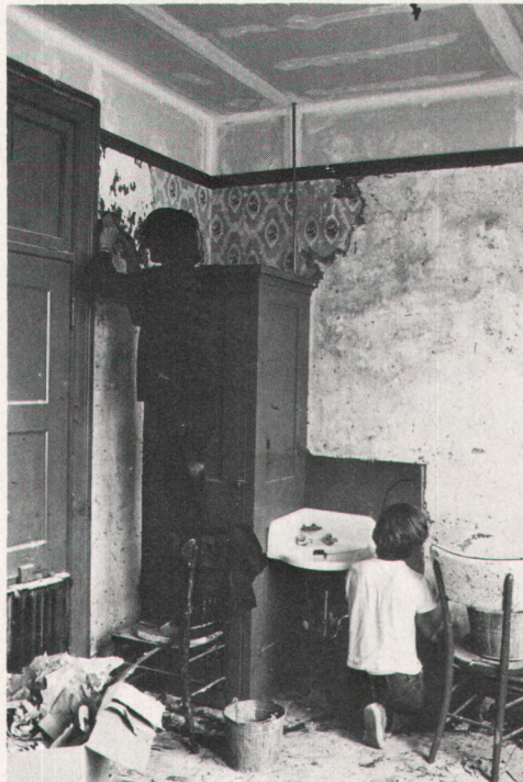
Volunteer Quaker high school students from the Bay area rehabilitate San Francisco's Imperial Hotel according to local CDC plans so that its elderly residents can continue to live there.
