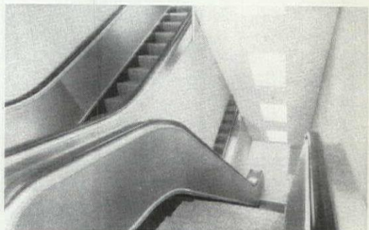
Sixteen Montgomery two-steps-level escalators in the core of the main building.
