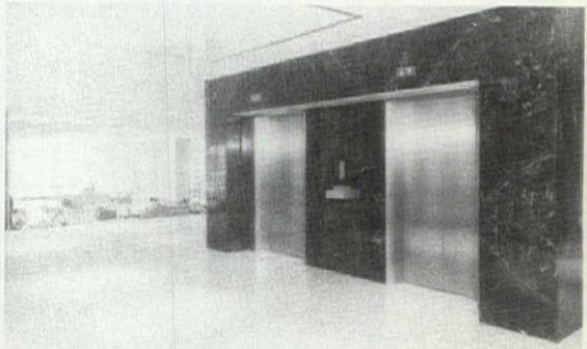
Express service to upper floors is provided by two high speed Montgomery elevators.
