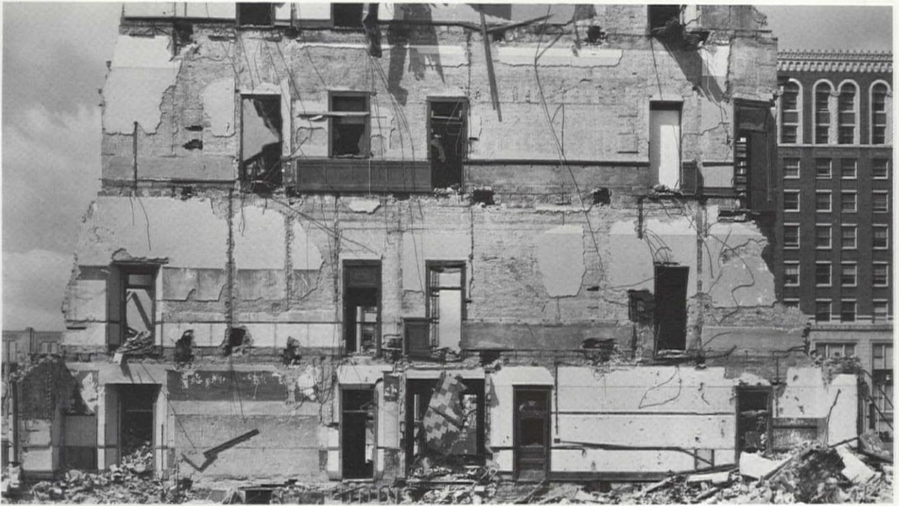
Restoration in progress: Careful stripping of plaster from interior walls reveals important features of original design.
